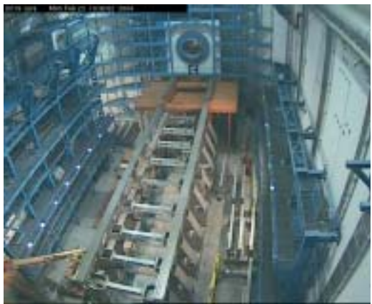
Status of the ongoing installation of the ATLAS detector in its underground cavern at CERN in Geneva, Switzerland. (From NY State participants include: BNL, Columbia, Albany and Rochester, etc.)
