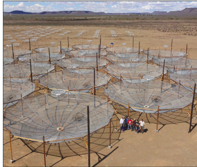
The start of construction on the HERA array. SKA South Africa, CC BY
