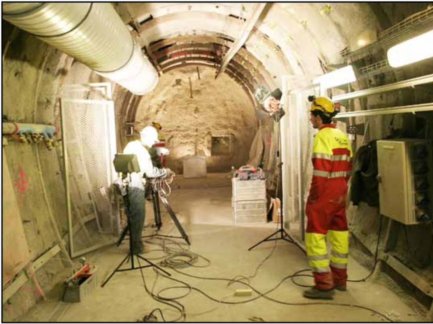
Subterranean experimental gallery of the Bure laboratory. Copyright 2006, Eric Sutre. Other photos of the facility can be found at www.andra.fr/index.php?id=itemmenu_phototheque_196_tout_1_1
