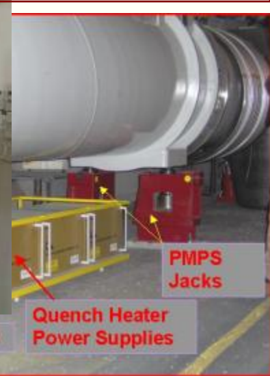
DAE's contributions installed in LHC Tunnel at CERN
