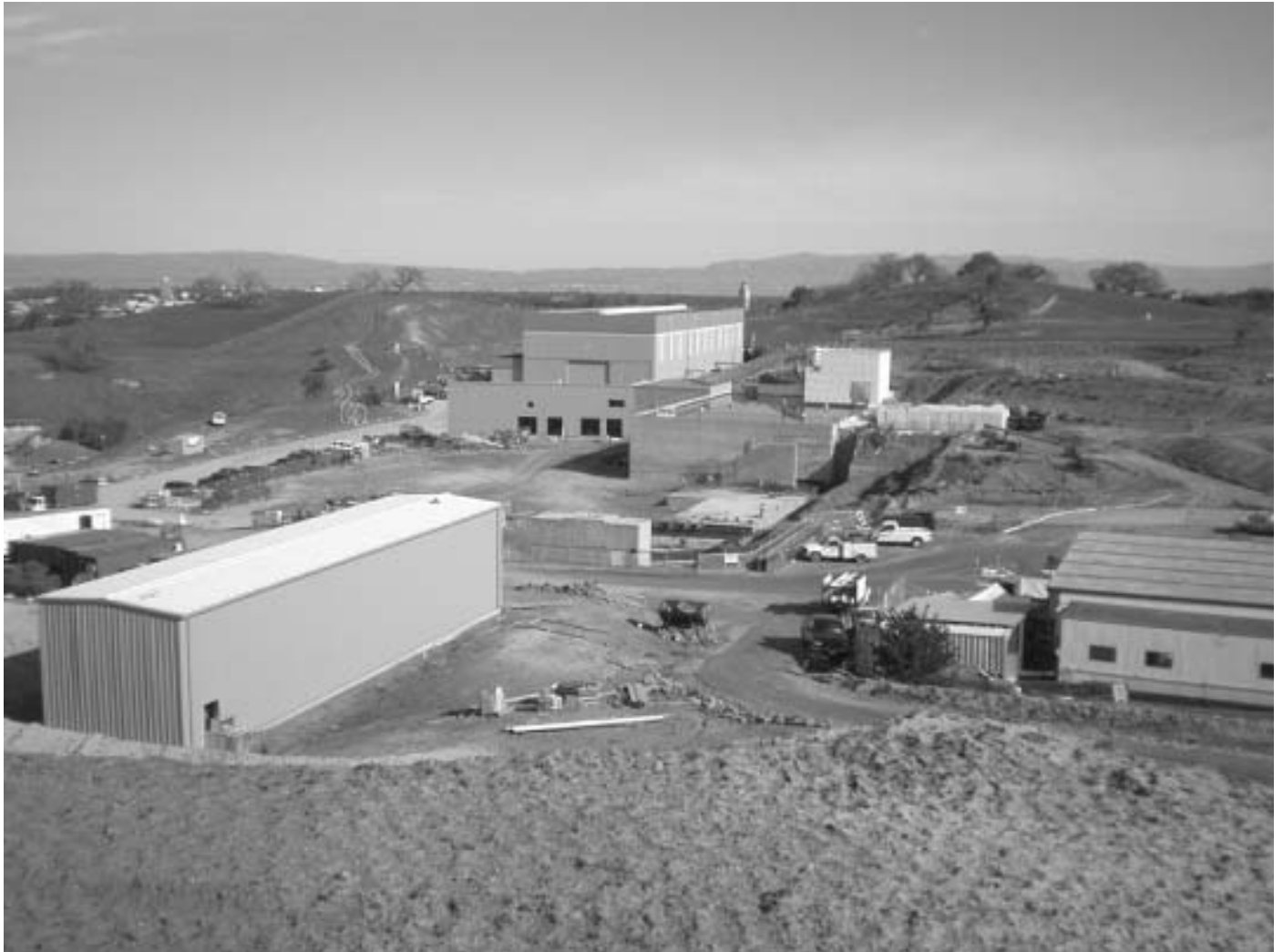
The undulator service building (left) and the new Near Experimental Hall (center) under construction on the SLAC site (facing east). Stanford University's Hoover Tower is seen in the background.
