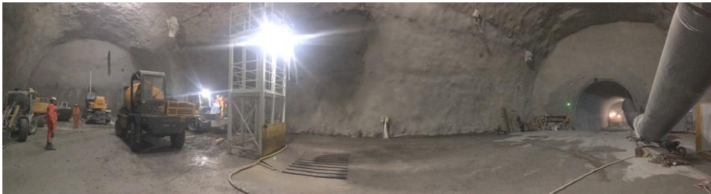
Figure 8. Base of the access shaft in Point 1 and start of the cavern excavation.
