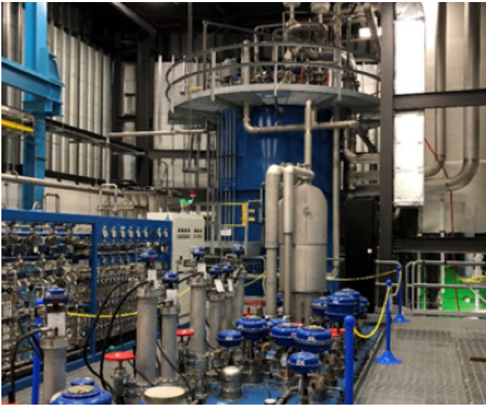
Figure 4. FRIB cryoplant operating at both 4 K and 2 K.
