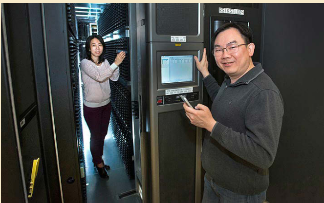
Figure 1: The RHIC and ATLAS Computing Facility, Source: BNL.
