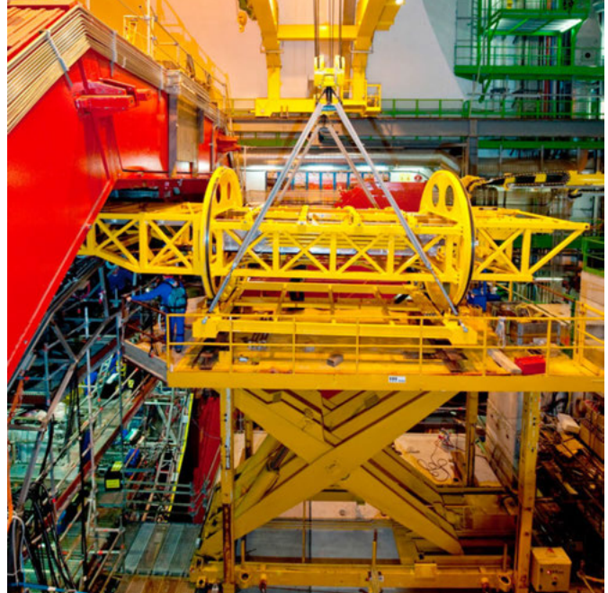
Figure 7.3: View of US-led ALICE ElectroMagnetic Calorimeter (EMCal) modules during installation in the ALICE experiment; one of the 10 EMCal modules, weighing over 7 tons, is being inserted.
